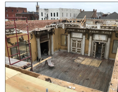
Looking southeasterly toward St. Mary Basilica, the roofless 2nd-story ballroom after cleanup but before reconstruction of the roof framing.
